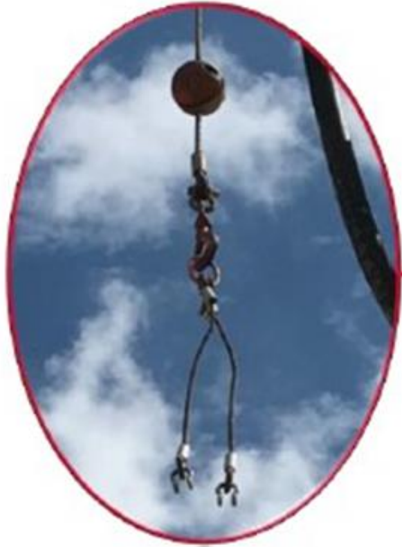
Failing Hoisting material
