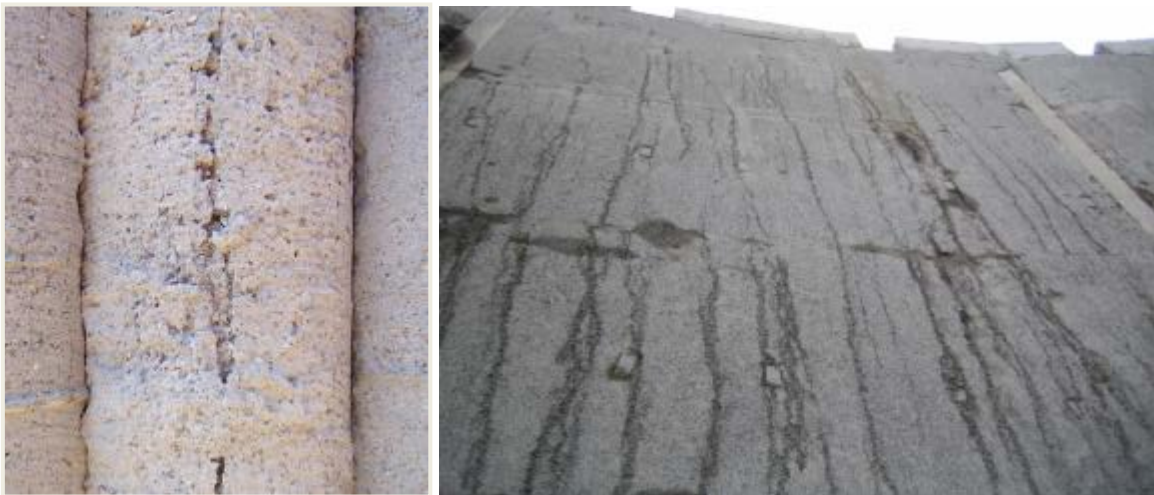
Figure D.3: Examples of channels running up the surface of a pile and a diaphragm wall
