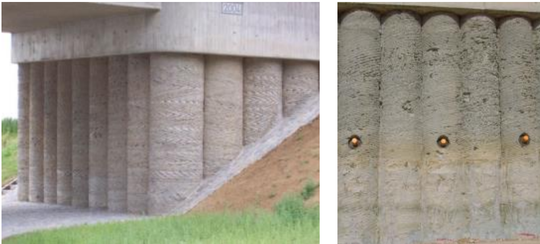
Figure D.1: Examples for piles with grooves, not affecting the minimum cover for durability
