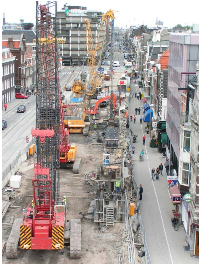
Fig 2: The Public are often walking on the other side of the site boundary without any protection.
