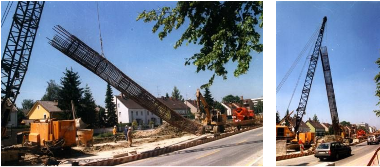
Fig. 1 A standard situation on construction sites in urban areas – featuring substantial accident potential
