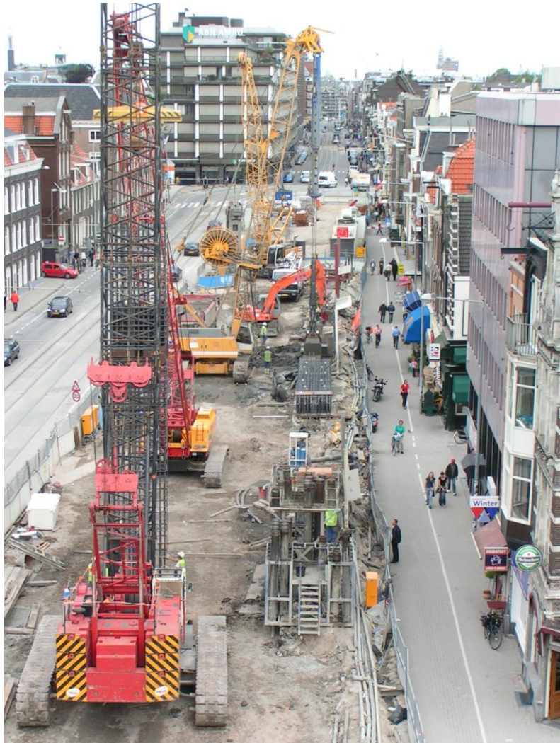
Fig 2: The Public are often walking on the other side of the site boundary without any protection.
